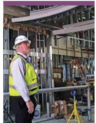
George Senerth, Executive Director of Facilities and Plant Engineering, looks over progress at the new wing.
